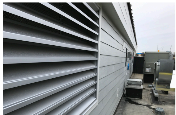
MECHANICAL & AIR FILTRATION
